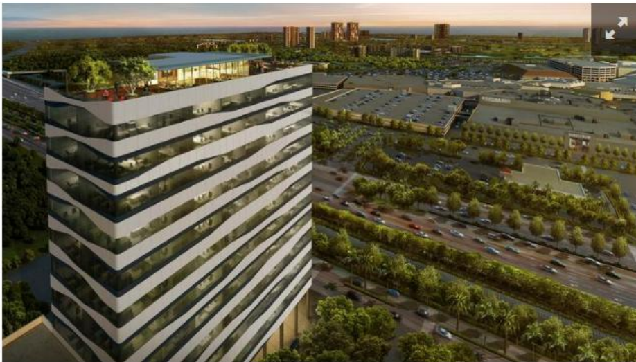
The 12-story Forum Aventura office condo is under construction at 19790 West Dixie... more
