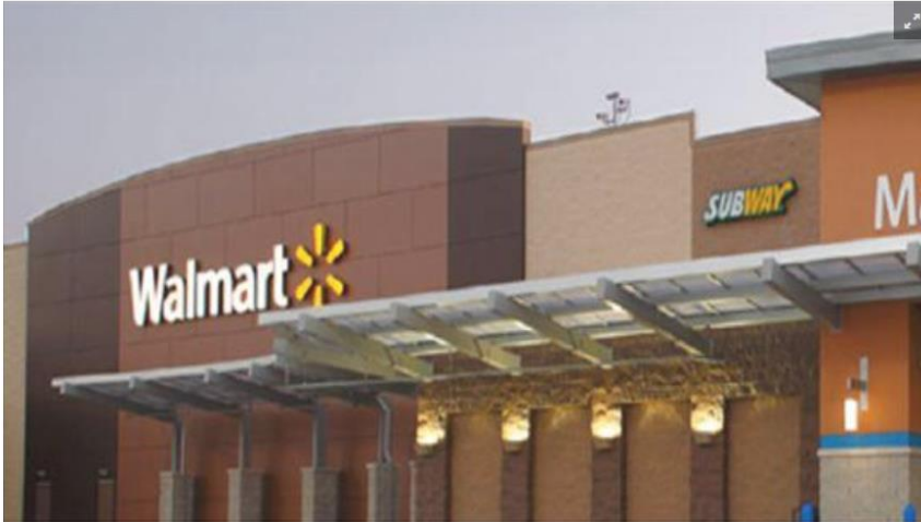
A Walmart Neighborhood Market is under construction at the southwest corner of Southwest 26th Street (Coral Way) and Southwest 147th Avenue in Miami-Dade County.
